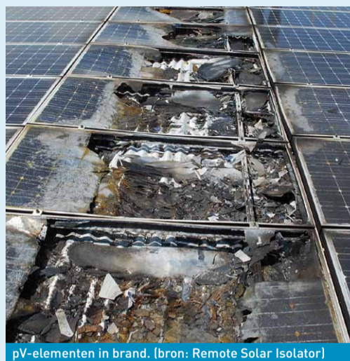
pV-elementen in brand. (bron: Remote Solar Isolator)
